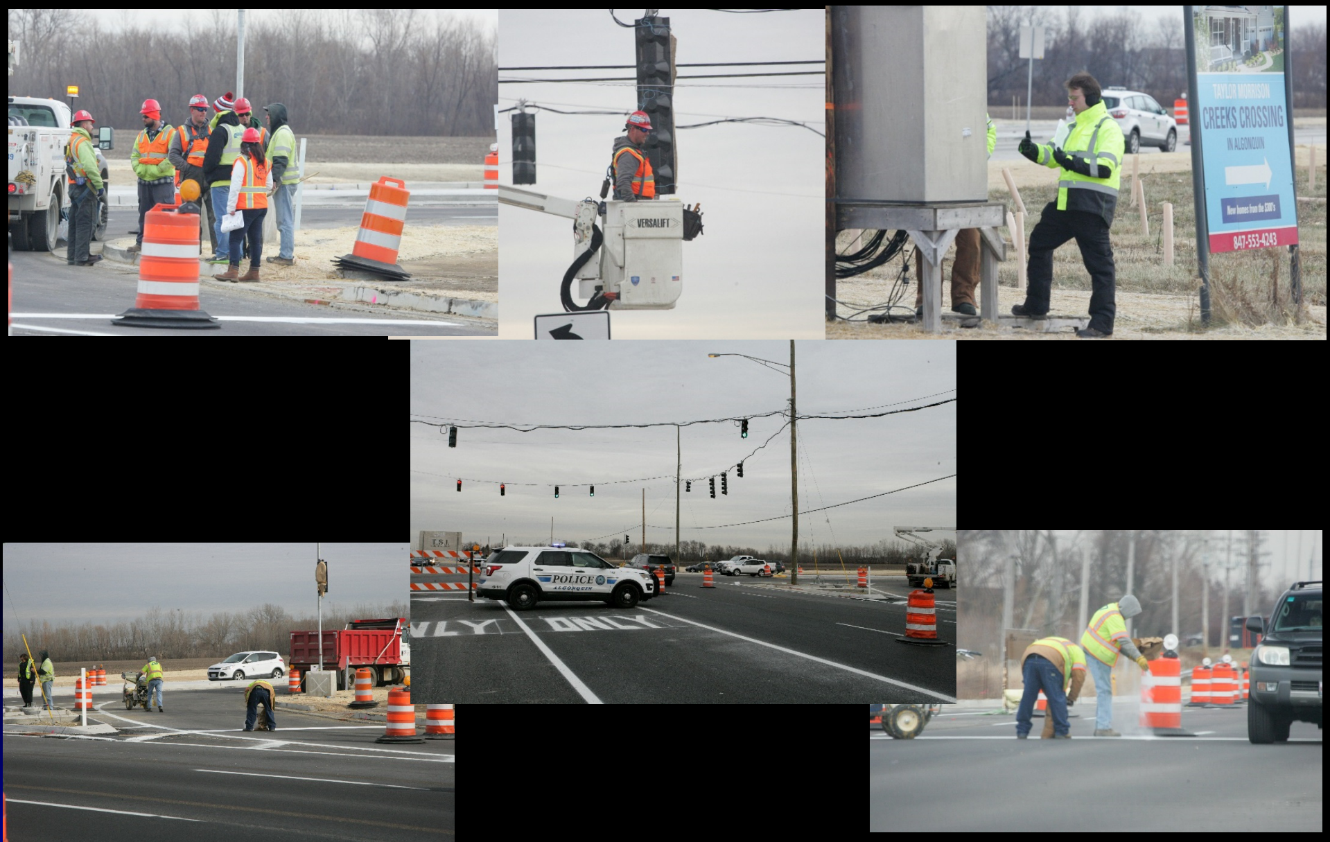
With a flurry of activity, including police presence for safety reasons, temporary traffic signals at Longmeadow Parkway and Randall Road are activated after roadway striping on Randall Road was completed
